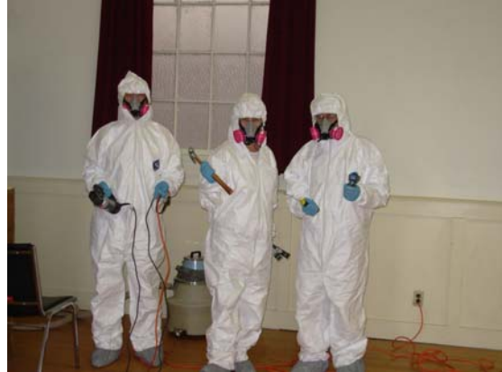
Caption: 1 Wilf, Lynn and Alewyn with chisels and hammers kitted up to remove gyproc and plaster from an area behind the stage at the request of engineers
